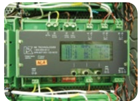
The LCD display shows the data points sent to a controller via network communication. The LEDs show proper network activity..
