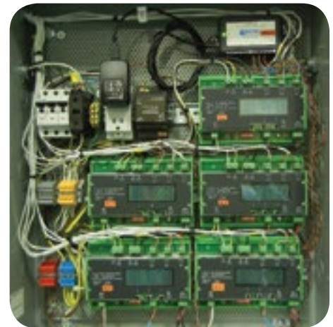
Five APN monitors monitoring the AC units at NK Technologies' factory in San Jose, CA..
